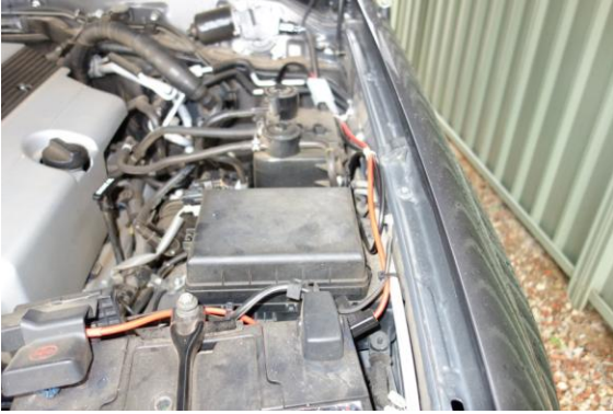
Picture showing the heavy duty DC cable red going to Battery + and negative to right body panel.
